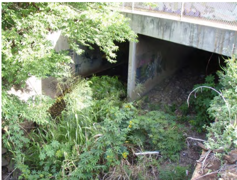
Figure 2 Exit of twin culverts beneath H1 Freeway above site. Left culvert (right side of picture) has 2-feet of rock rubble over bottom. Left culvert is clear and drops about 3 feet to eroded stream bed at exit.
