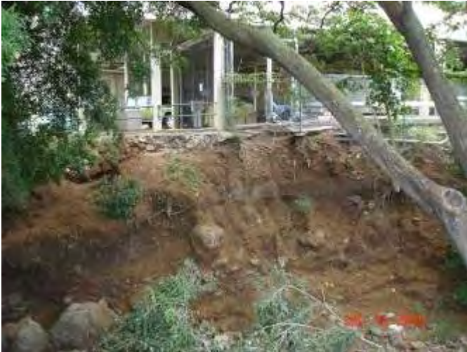
Figure 8. Aiea Shopping Center Bank Erosion at Station 305+23 to 305+51.
