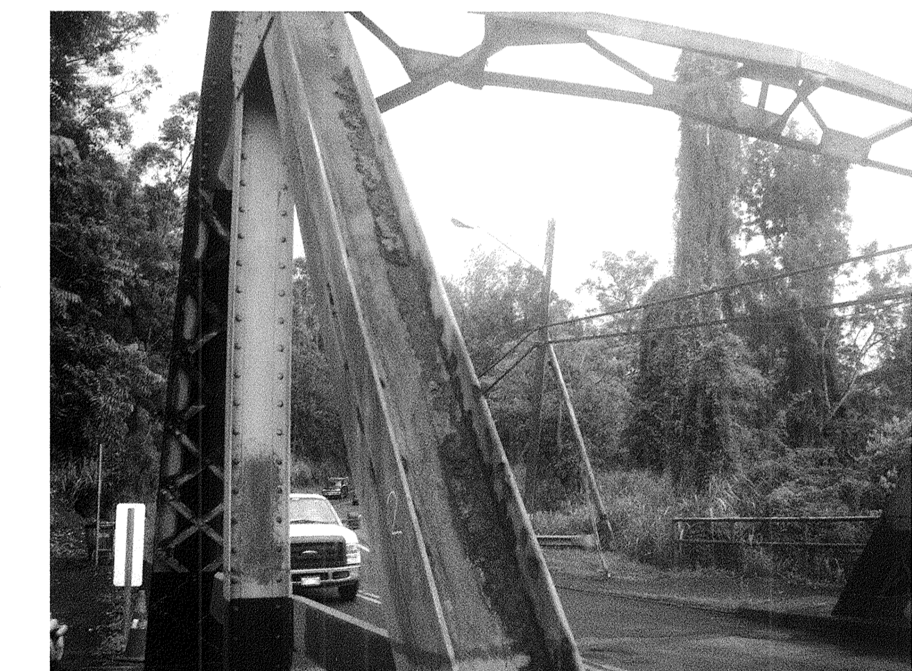
4 EXISTING WEB MEMBER DETERIORATION S5.20 | S5.20
