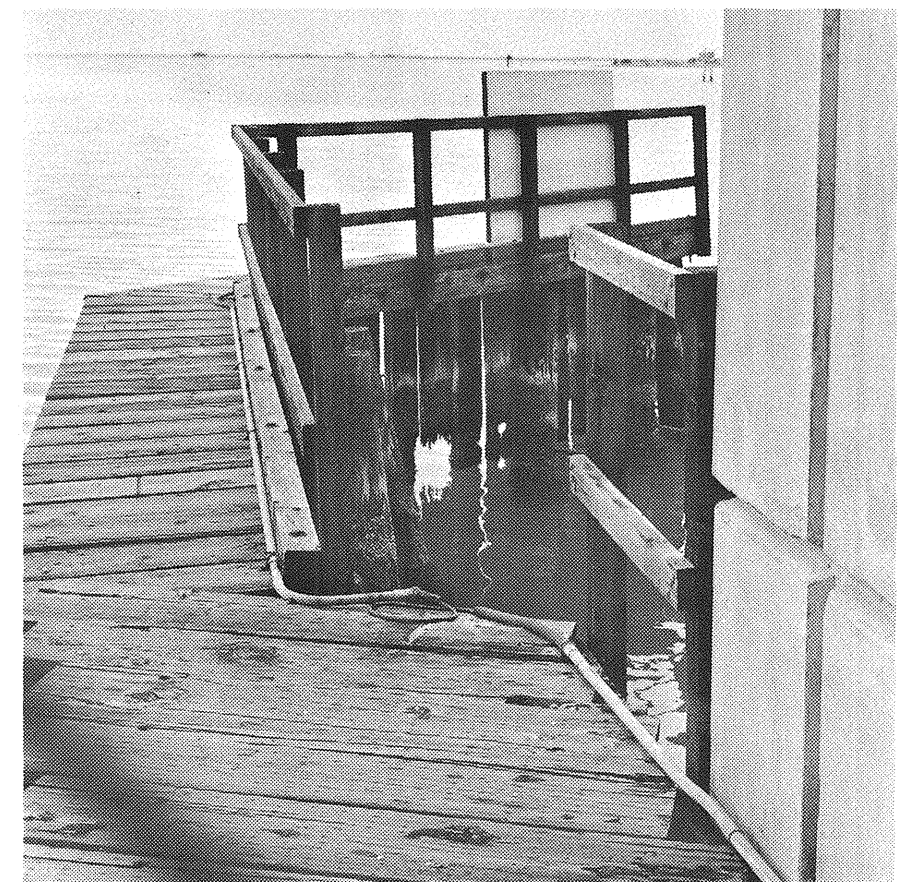
NORTHWEST PIER WIRING (7)
