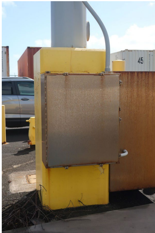
Photo 4: Pole B3 - Communications Equipment Cabinet
