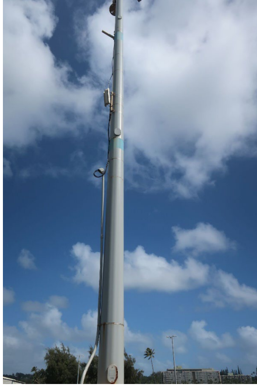
Photo 3: Pole B3 - Antenna and Transceiver
