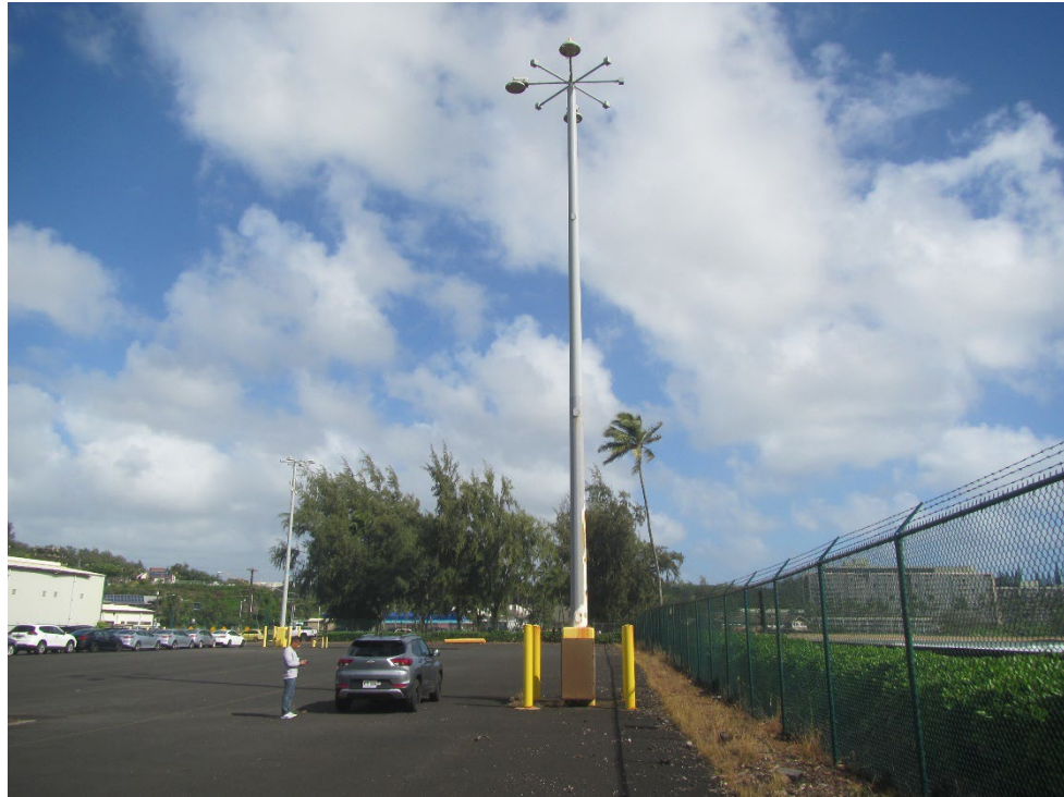
Photo 1: Typical Pier 1 Pole (Pole B2 Shown)
