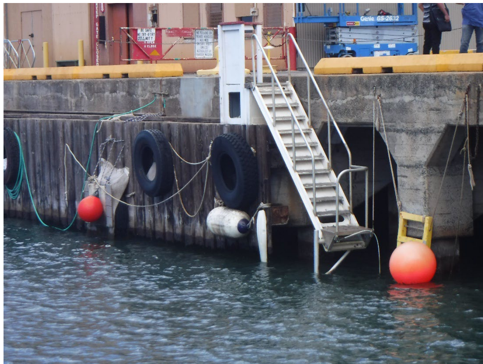
Photo 4: Stairs to be Replaced
