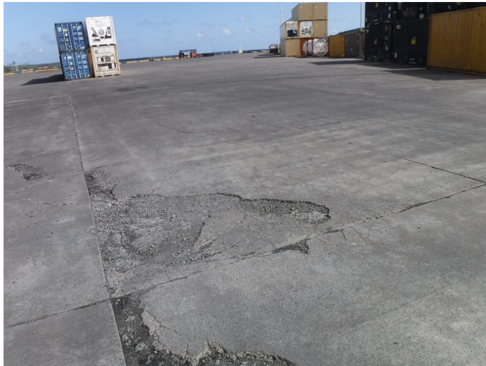
Photo 2: Typical Damaged Concrete Pavement
